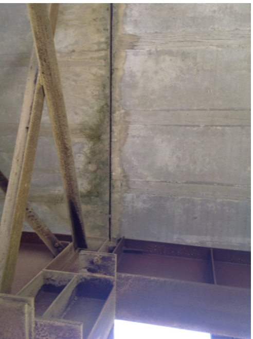
panel damage at jumpspan
